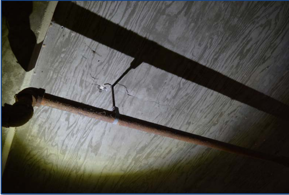
Photograph No. 5: Sprinkler piping in the basement is rusting and will need sanding and painting soon.
