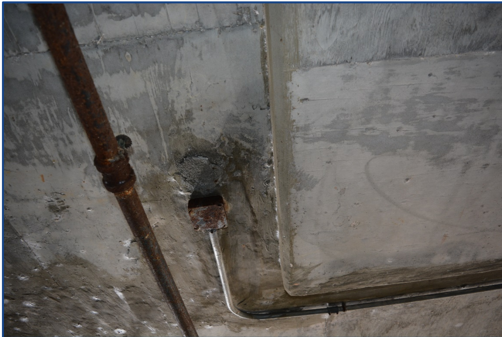
Photograph No. 4: The sprinklers in the unconditioned space have a 40-year design life. Sprinkler heads need replacement.
