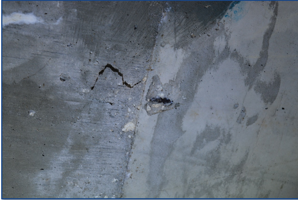
Photograph No. 7: The garage ceiling needs to be repaired when defects occur.
